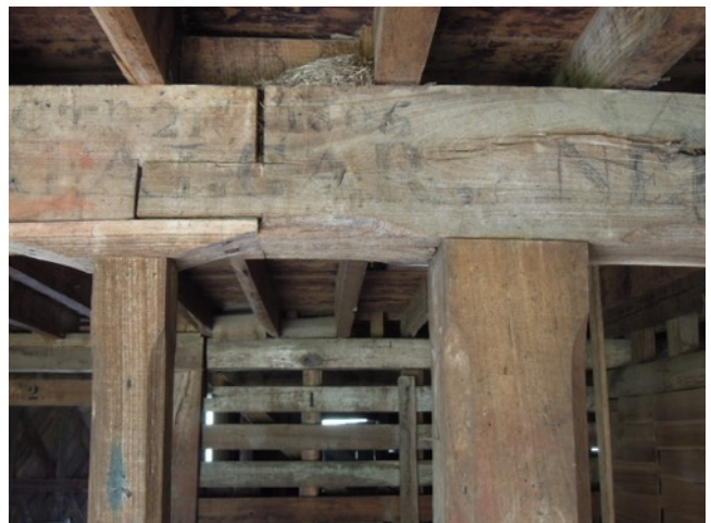
Evidence of structural alteration. Woolmers Woolshed
