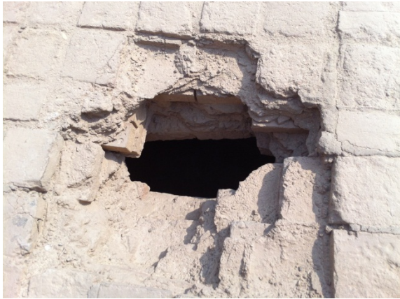
[Photo Caption: A manhole sized crack on the top of a wall at the Abbasid era Bab Al-Wastani (The Middle Gate) in Baghdad. The hole was clearly used to penetrate the ancient wall. Credit: Dr Benjamin Isakhan, 2012.]
