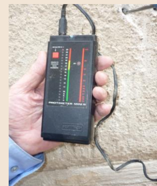
Measuring dampness in walls Protimeter reading 100%
