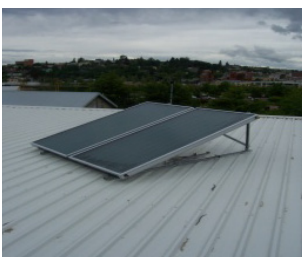
North split solar system
