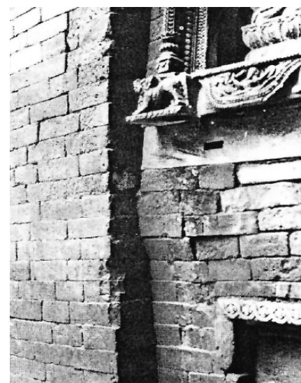
Fig. 7. Local bulging of brickwork beneath a niche. The panel of brickwork on the left is the other end of the panel shown in Fig. 3. The decorative timber of the door sill (lower right) has decayed severely, and the small vertical piece has been replaced with brick tiles.
